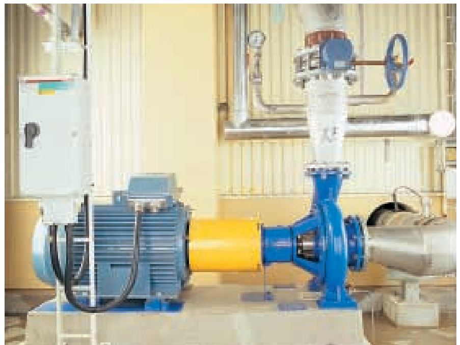
Installation in the chemical industry, Akzo Nobel, Bohus in Sweden. The pump is mounted on a concrete foundation.
